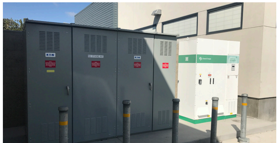
Energy storage system at Earl Warren Middle School
