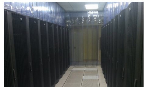
Data Center, Canton, MA
